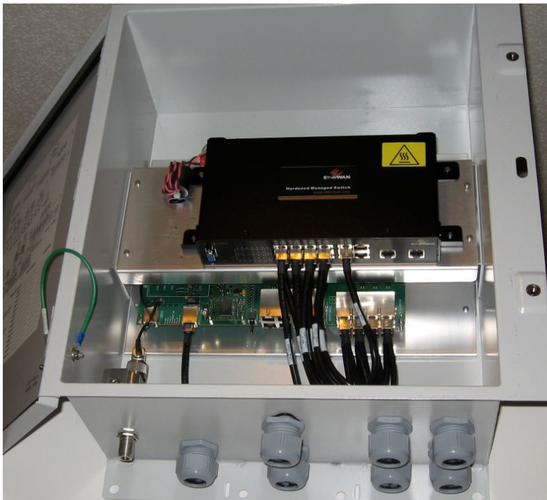
Figure 14 CMM4 (Cabinet with switch)
