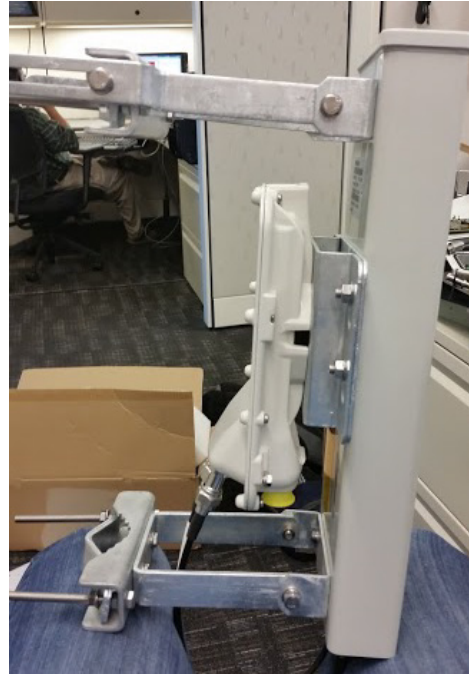
Figure 43 Completed AP and antenna assembly
