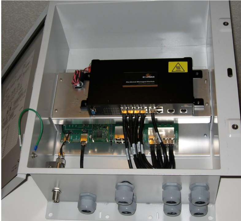
Figure 26 CMM4 (Cabinet with switch)
