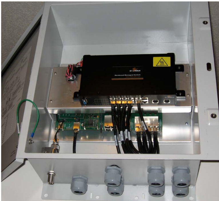
Figure 36 CMM4 (Cabinet with switch)
