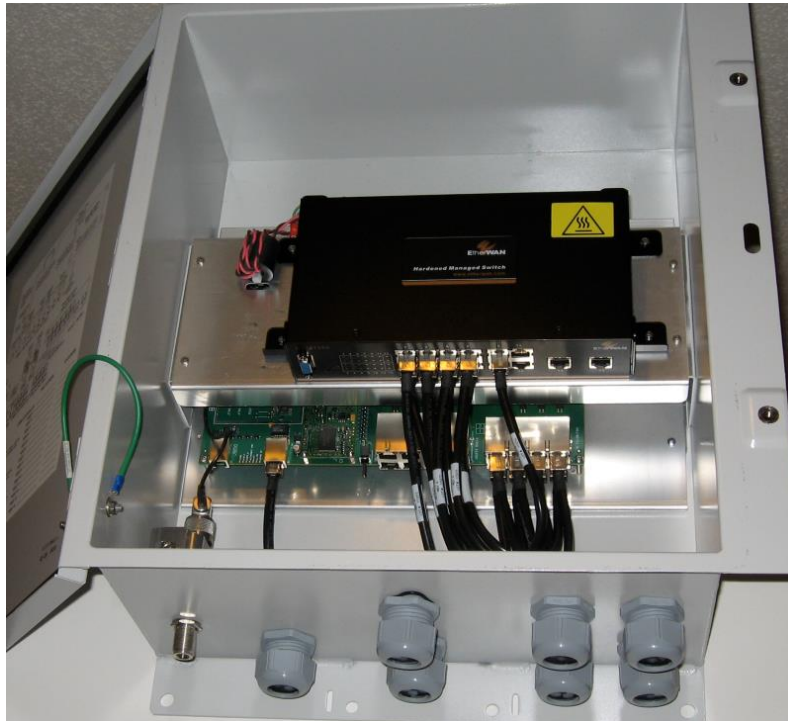
Figure 26 CMM4 (Cabinet with switch)
