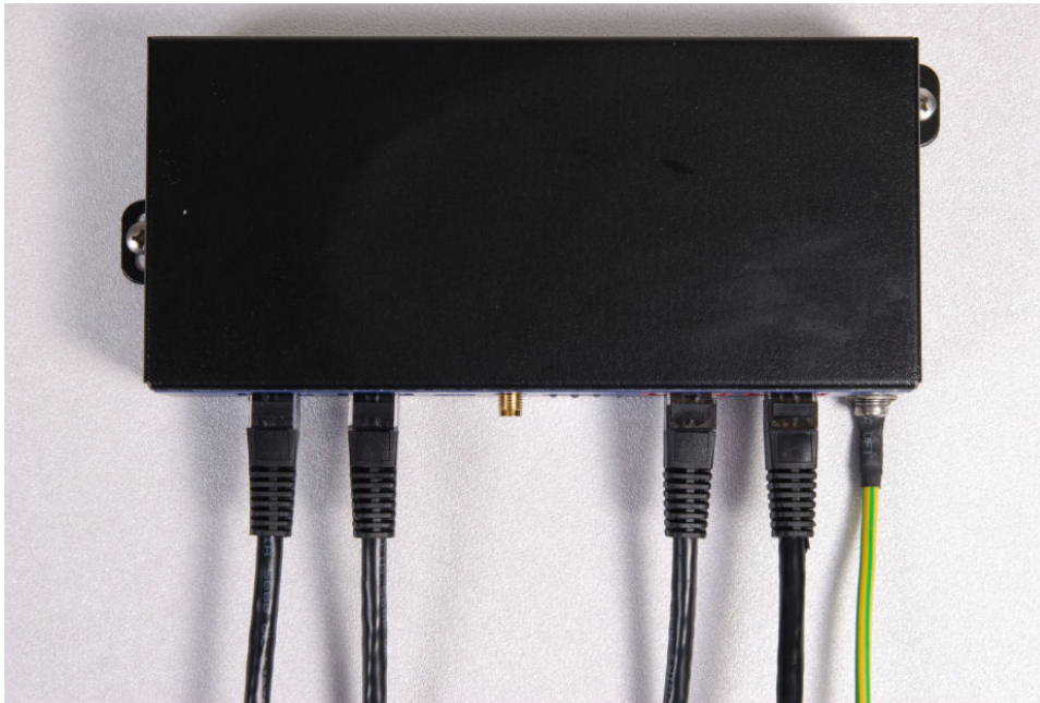
Figure 97 PTP-SYNC mounted on a wall
