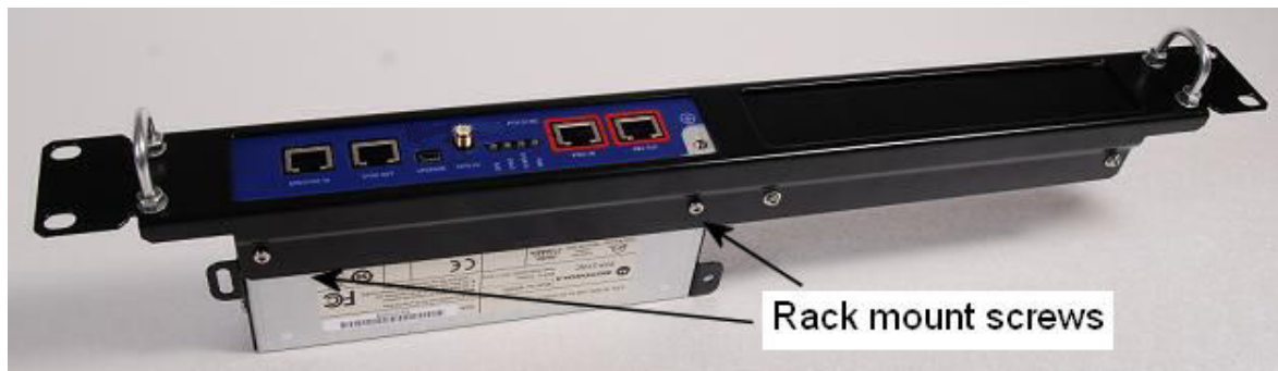
Figure 96 PTP-SYNC mounted in a rack
