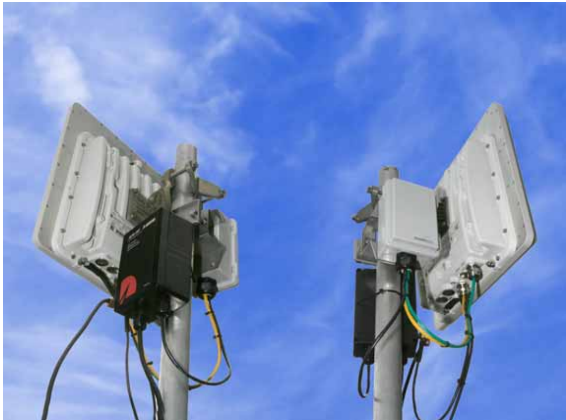
Figure 128- GPS Synchronization Unit Complete Installation
