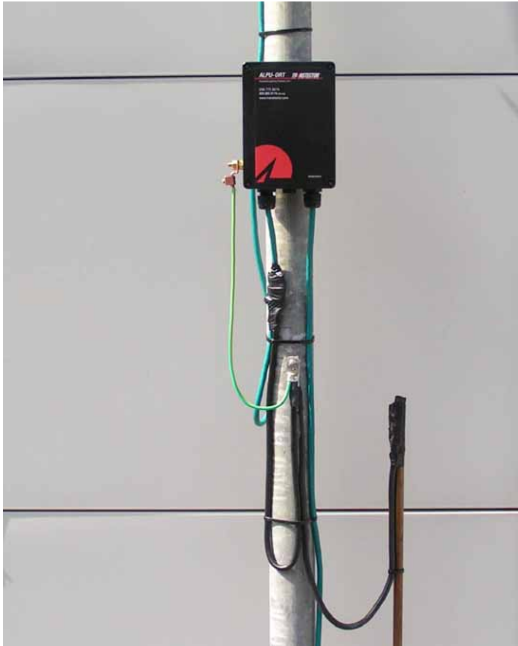
Figure 111 - Lower Grounding Configuration
