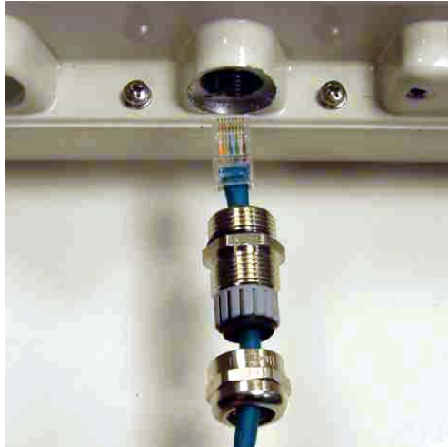
Step 1: Assemble the cable as described in 5.7.1 above
