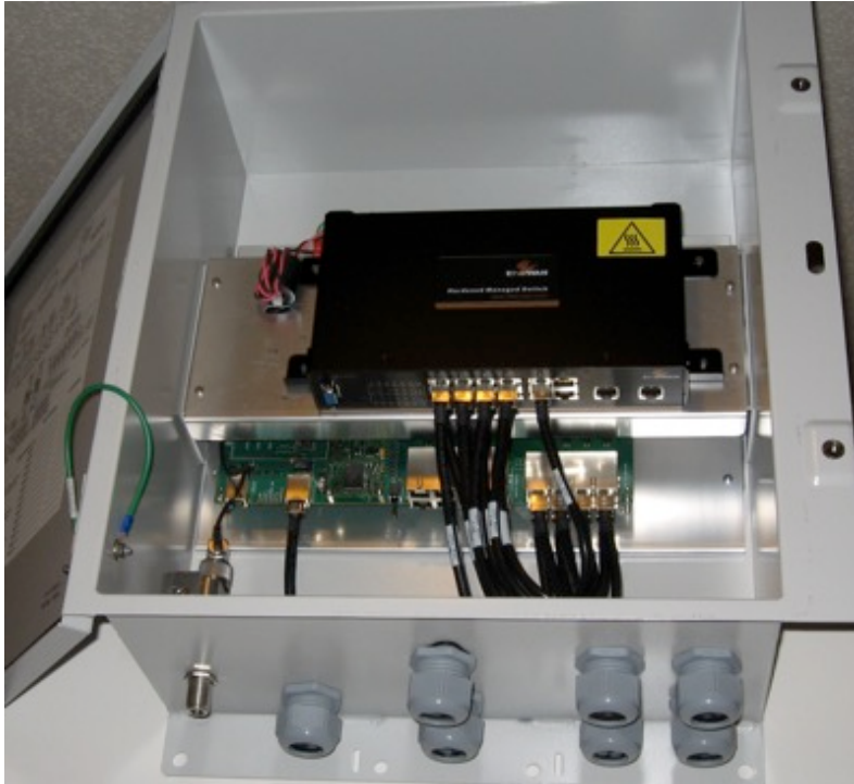
Figure 17 CMM4 (Cabinet with switch)
