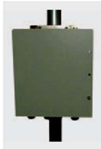
Figure 28 Pole mounted CMM3
