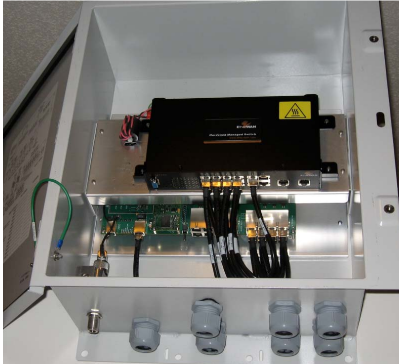
Figure 26 CMM4 (Cabinet with switch)
