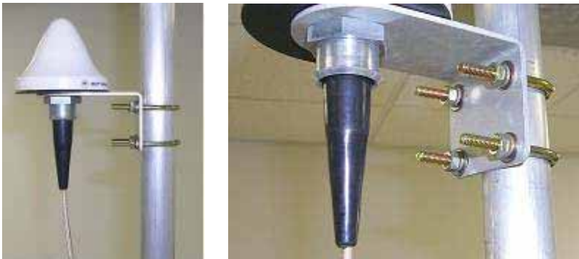
Figure 43 GPS antenna mounting
