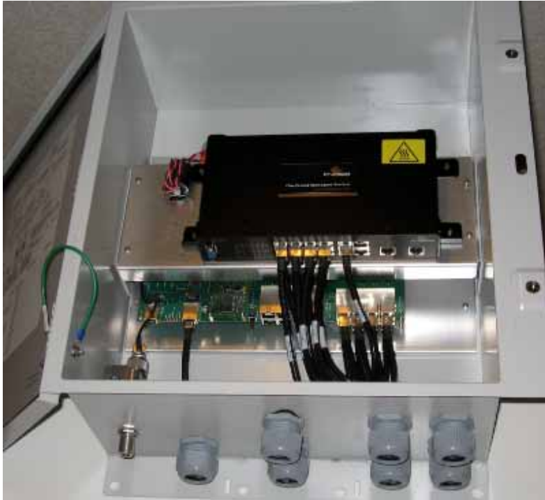
Figure 40 CMM4 (Cabinet with switch)
