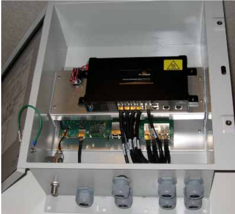
Figure 40 CMM4 (Cabinet with switch)
