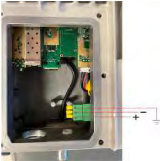
Figure 10 : 3 GHz cnRanger 210 RRH DC power cable
