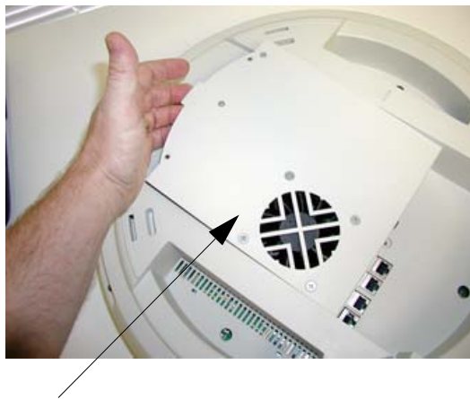
Access panel (with power supply and fan)
