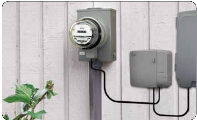
Our RFOG and GPON Fiber Power Systems provide the same reliability as our HFC systems with added features including outdoor access to batteries and multiple configuration options.
