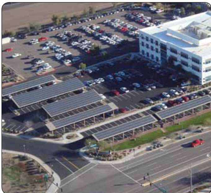
Grid-Tied Solar Power can help minimize operating expenses and reduce your carbon footprint. (153kW Grid-Tied system in Phoenix, AZ)
