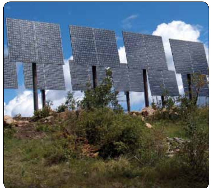
Off-Grid Solar and Hybrid Power Systems can provide the necessary redundancy for critical loads and help extend network signal to remote areas. (1kW Off-Grid Hybrid Power System in Southwest Colorado)
