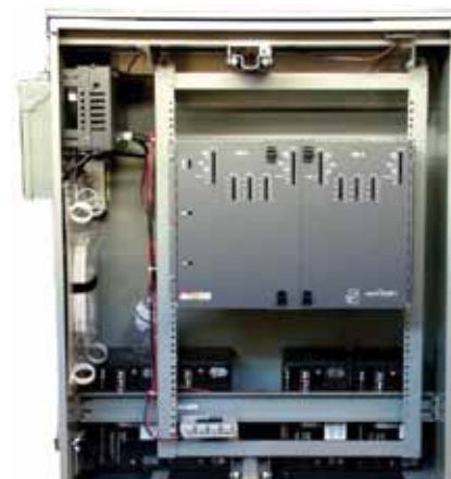
Shown with FTTx actives installed, 19" swing rack, 50Ah AlphaCell batteries, AC and DC distribution, Fiber management and 300W power supply
