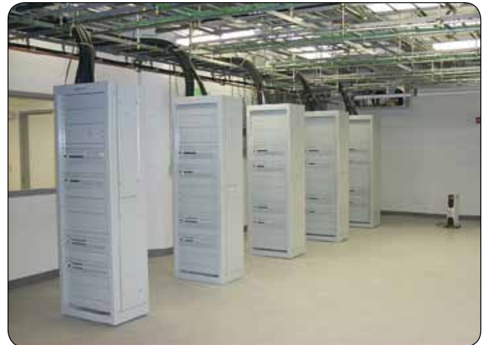
Electrical system capabilities up to 1200Amps.
