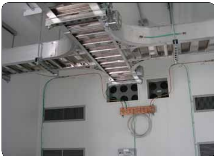
Custom wall framing allows units to be pre-wired and equipment-ready upon arrival.
