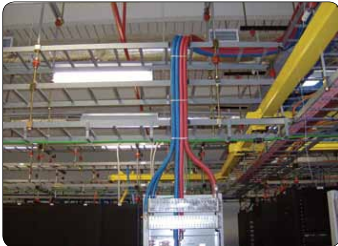
Pre-wired and equipment ready.
