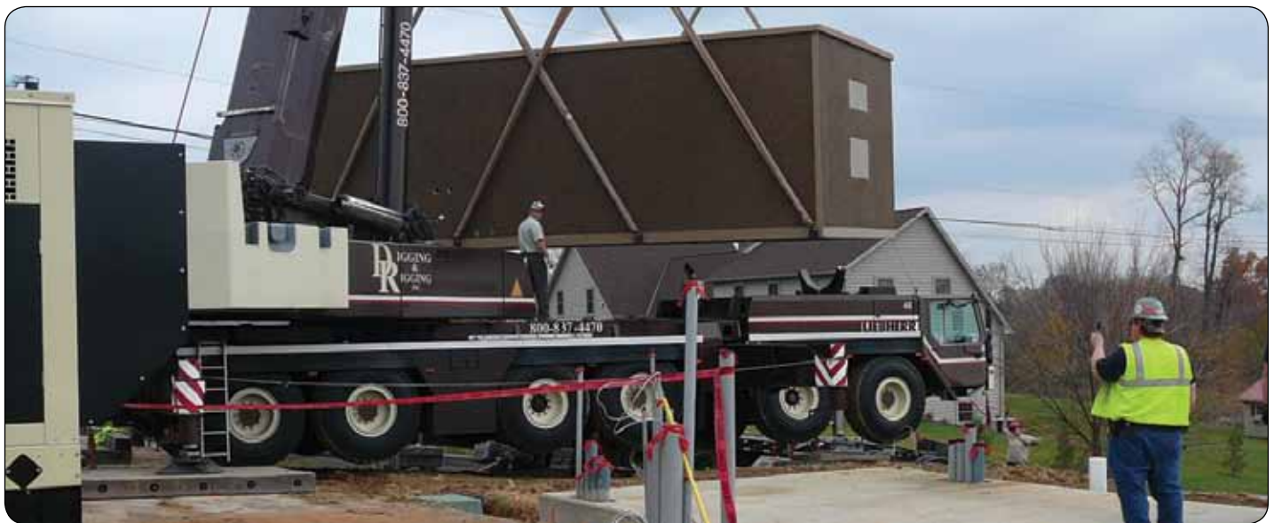
Alpha project managers will complete all site surveys, geological testing, engineering drawings and building permit applications. Our nationwide network of contractors and project managers then coordinate the entire implementation on-site, from concept to commissioning.
