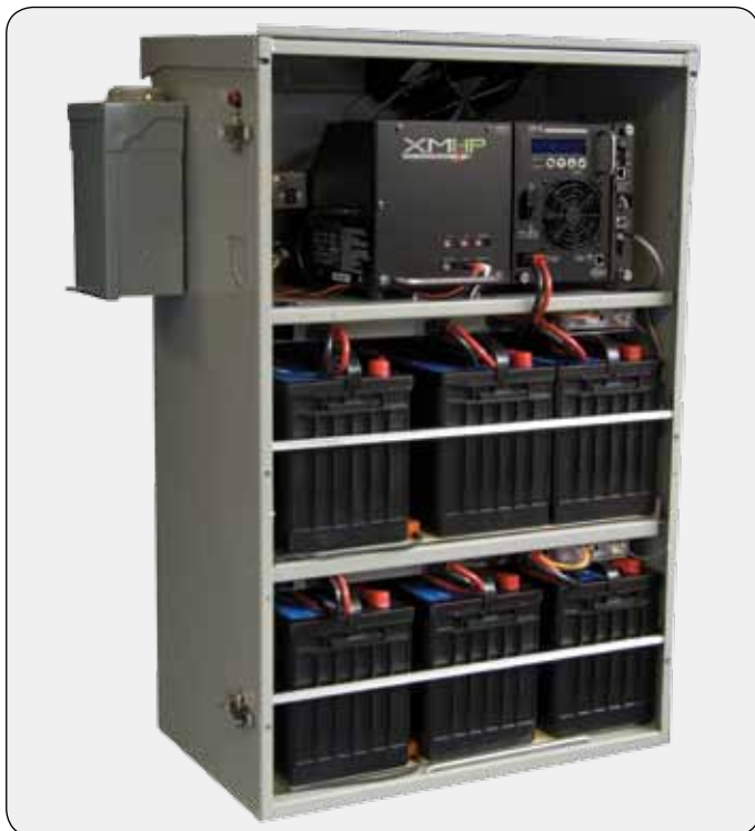
High performance outside plant systems include multiple power supply, enclosure and battery options, as well as a full line of system accessories for climate-specific applications to provide extended runtimes and protect your powering investments.
