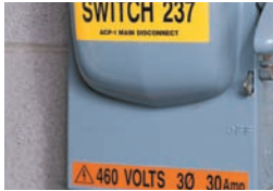
Panel & Switch I.D.
