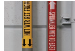
Pipe & Valve ID
