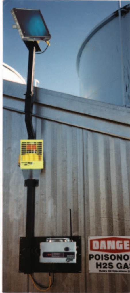
Remote Sensor mounted on wall.
