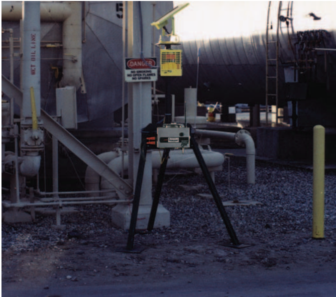
Sensor Mounted Under Pipeline
