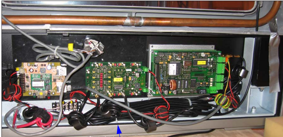
Cables are dogbone wrapped and routed along the bottom
