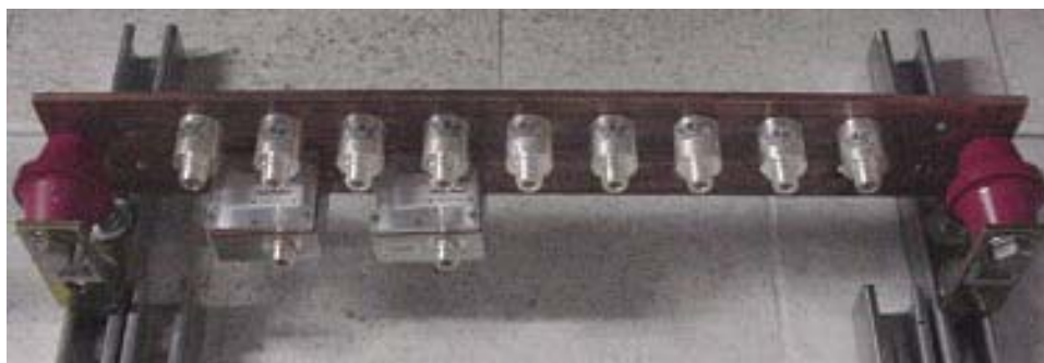
Figure 12: Surge Protectors in Buss Bar (Non-TTA system)
