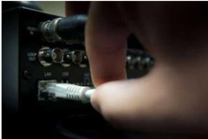
Figure 31 Ethernet Cable to DVR Unit
