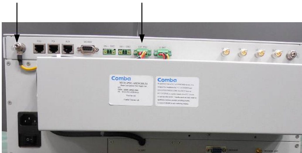
Figure 10: Backup PSU Installation 2
