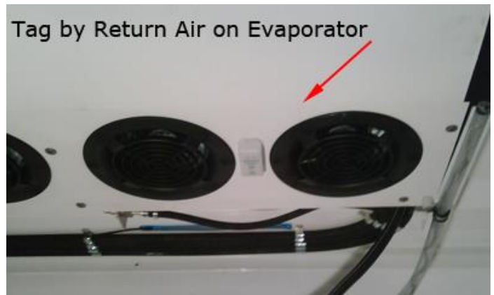
Temperature Tag located next to the Return Air duct
