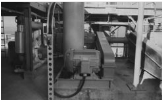
Control Cable Entering Pushbutton and Power Cable Entering Motor Terminal Box from 6 Inch Channel Cable Tray System (Bottom entries provide drip loops to prevent moisture flow into enclosures.)
