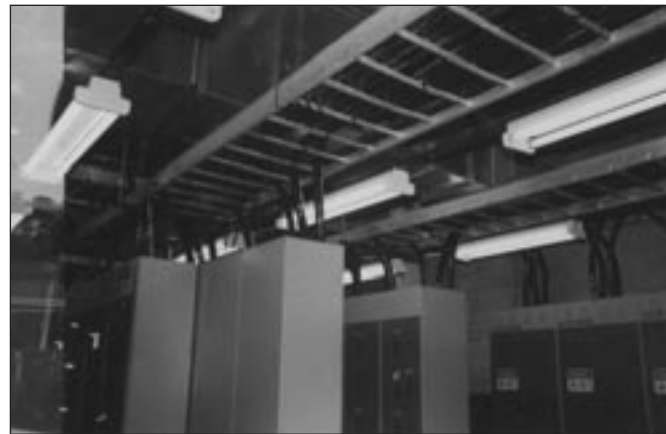
Cables Entering and Exiting Motor Control Centers from Cable Tray Systems.
