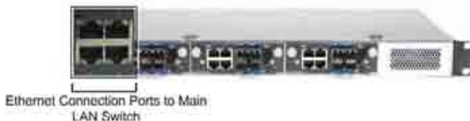
Figure 6-2. CEM LAN and Fiber Connection Ports
