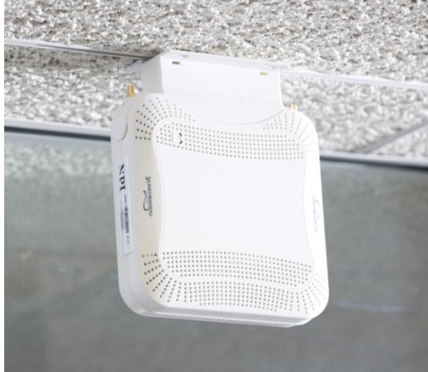
Figure 5-3. VAP Mounted Vertically on Ceiling
