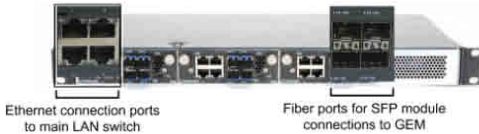
Figure 5-1. CEU Ethernet and Fiber Ports
