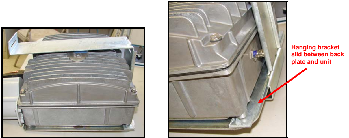
Figure 47 – Bracket attached to CT Backhaul-Point
