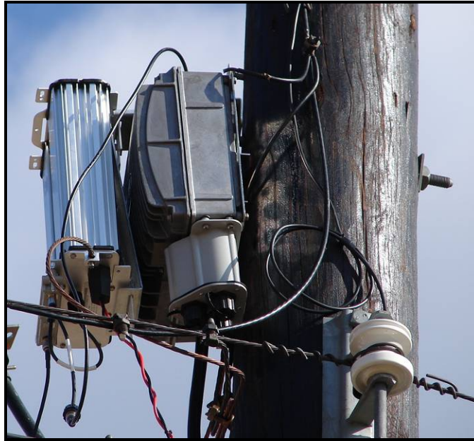
Figure 50 – Gateway-Bridge installed with CT Backhaul-Point
