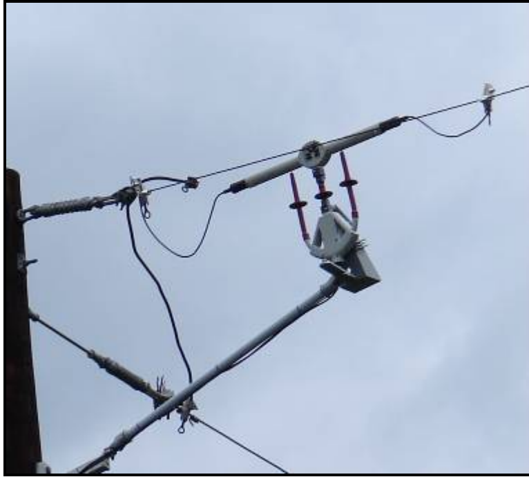
Figure 19 – CT Coupler Hung Incorrectly
