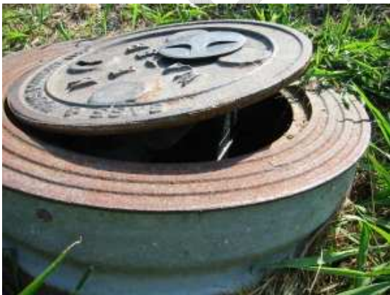
Example of a BAD Sensor-end Installation. What is wrong here? _____
