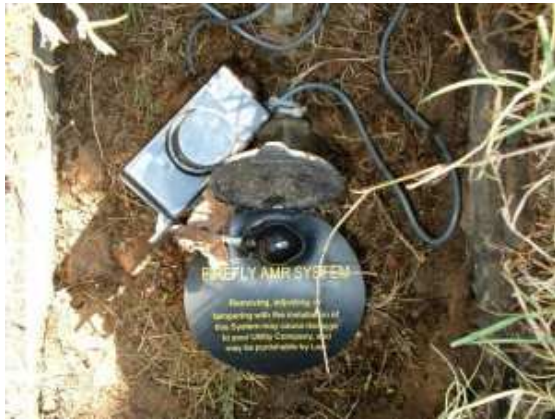
Example of a GOOD Sensor-end Installation.
