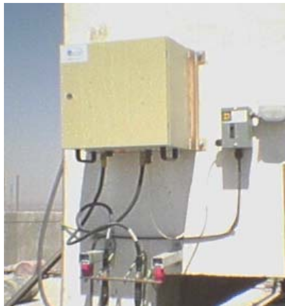
Figure 45: iDEN Repeater – Typical Outdoor Installation
