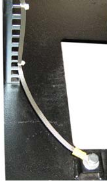
Figure 9. Final Grounding Connection
