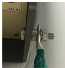
Figure 47 Remote Ground Connection
