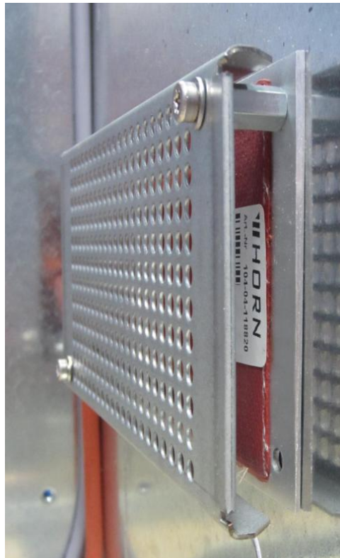
Fig. 72: View of cabinet heater
