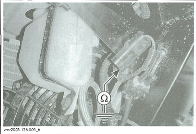
FAN GROUND CIRCUIT CONTINUITY TEST (BKACK WIRE)
