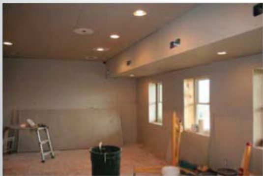
The room during the drywall stage, with a DriCore subfloor, a long soffit hiding the ductwork, and recessed in-ceiling can lights.
