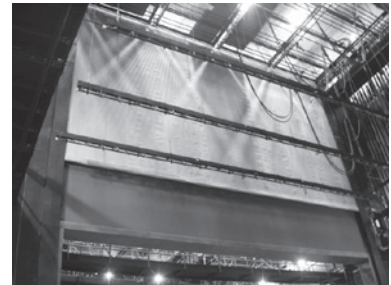
Straight Lift Fire Curtain
