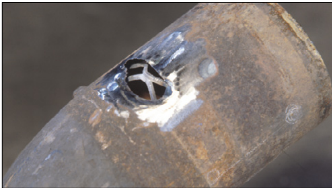
The wire mesh reinforces the repair area and forms a mechanical backing for the epoxy.
