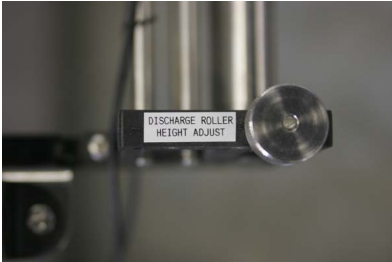
Controls and Connections
