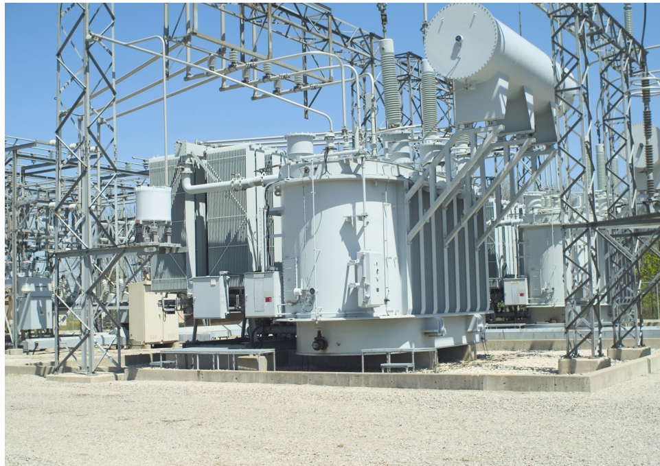
Three-phase transformer bank used for power distribution.
