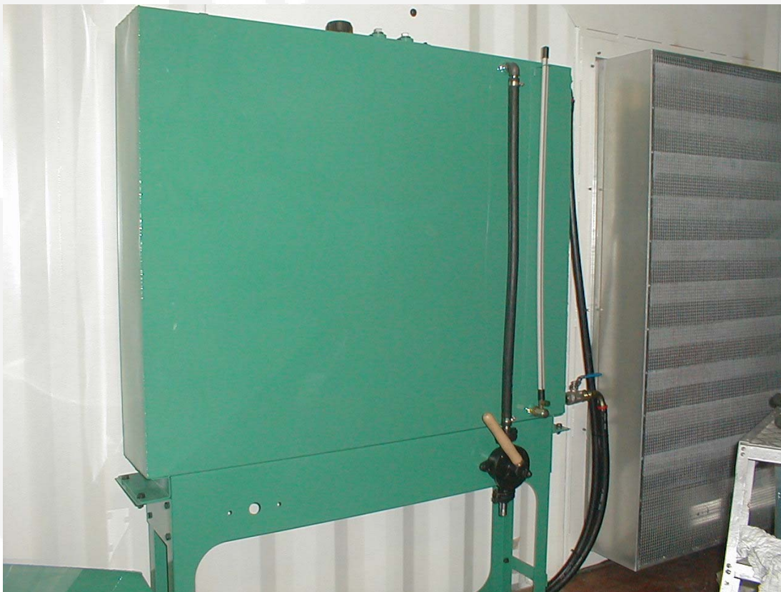
Figure 6-3 40S PowerBox fuel tank positioned behind alternator against wall
