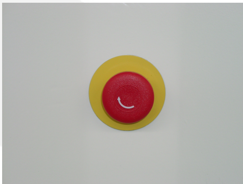
Figure 6-8 Emergency Stops (E-stops) are fitted next to the service doors.
