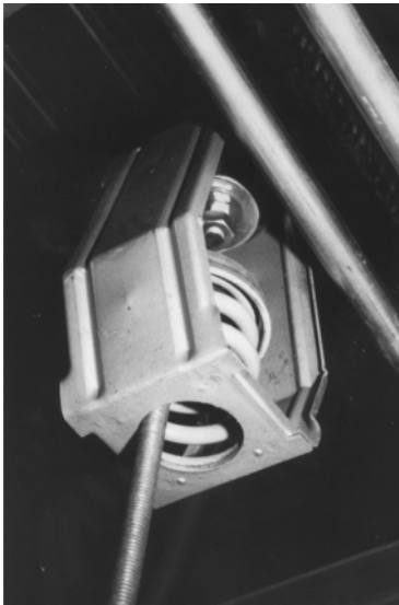
Figure 7-8 Faulty spring hanger installation with hanger rod touching the hanger box. This allows pipe vibration to bypass the spring and enter the building structure above.
