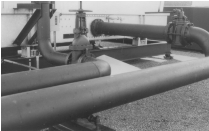
Figure 8-18 Incomplete vibration isolation at cooling tower. Even though the tower is isolated, the condenser water pipe supports are mounted rigidly to the roof. This allows some tower vibration to enter the roof structure.
