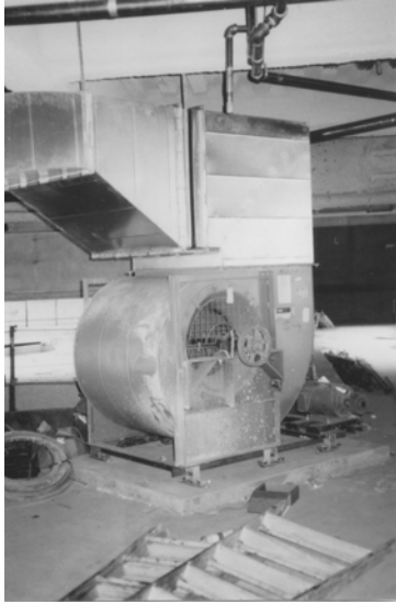
Figure 8-2 Example of poor fan discharge duct design. The mitered elbow with turning vanes and steep transition downstream of the fan outlet cause fan instability and accompanying noise and rumble. A better installation would have used a horizontal discharge fan with fewer downstream fittings.
