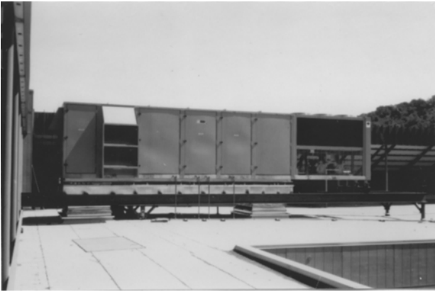
Figure 8-6 Excellent rooftop package unit installation; the unit is resting on spring isolators and an elevated frame, thereby avoiding contact with the roof.
