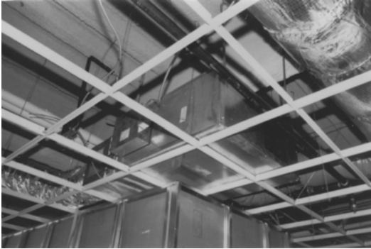
Figure 8-7 Improperly installed fan-powered variable-air-volume unit. The unit is resting on the ceiling grid. This allows vibration to transmit directly into the partition below. The partition then acts as a sounding board, radiating noise into the occupied space.
