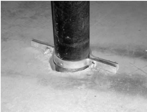
Figure 7-10 Pipe risers without vibration isolation. The pipe clamps transmit pipe vibration to the slab.
