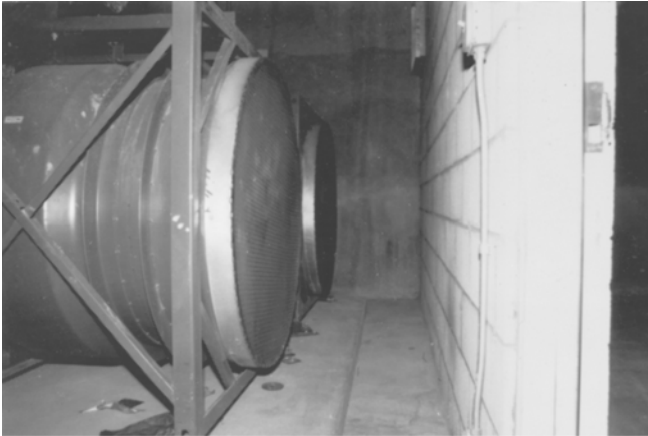
Figure 8-12 Vane-axial fan intakes too close to wall. Airflow through the restricted area between the fans and the wall causes turbulence, surging, and rumble.
