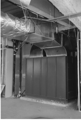
Figure 2-20 Plenum AHU with supply ducts attached to the top of discharge plenum.
