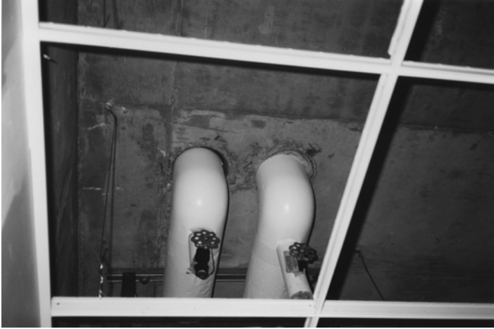
Figure 8-21 View of pipe penetration from below roof. The pipe on the right is contacting the left edge of its penetration. This installation allowed pipe vibration to excite the roof slab, which radiated the energy as noise.
