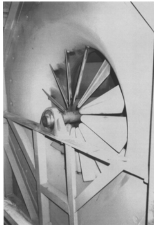
Figure 2-51 Nested inlet vanes obstruct airflow.
