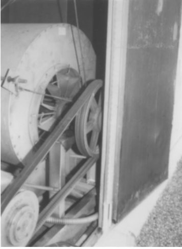
Figure 8-5 View into the fan section of a rooftop unit; the tight cabinet clearance and airflow obstructions at the fan inlet cause excessive turbulence, pressure drop, and noise.
