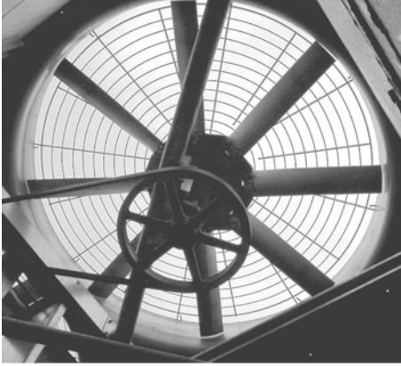
Figure 3-5 View of “standard” cooling tower induced-draft fan.
