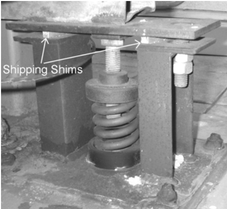
Figure 7-7 Short-circuited floor mount isolator whose shipping shims have not been removed.
