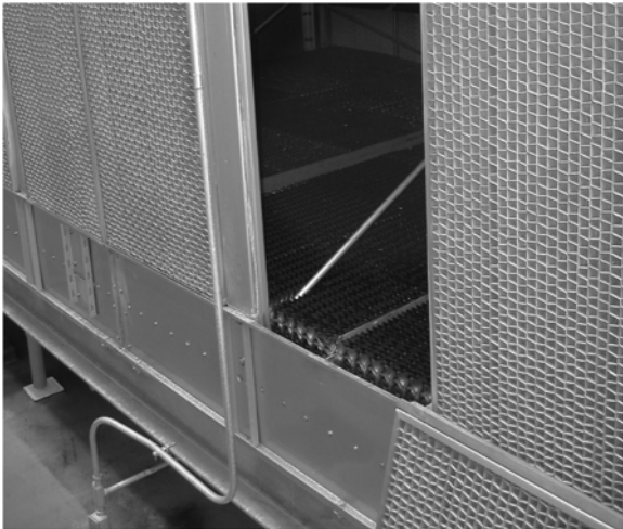
Figure 3-9 Honeycomb water basin silencers installed several centimeters above the water surface to reduce the velocity of the falling water before it hits the basin.
