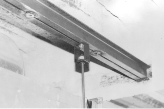
Figure 7-5 Overloaded spring hanger.
