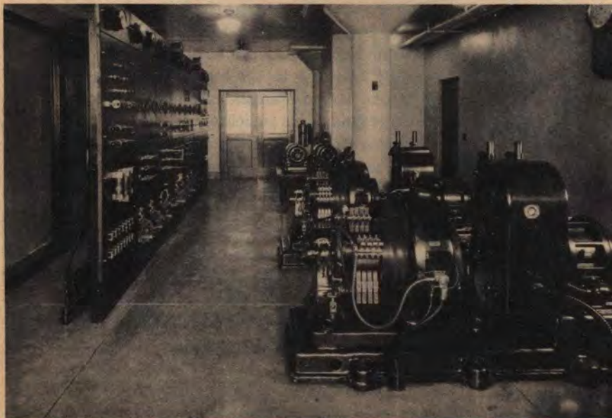
TYPICAL REPEATER STATION POWER PLANT
