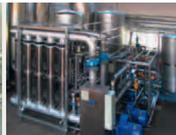
Ceramic filtration plant
