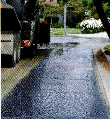
Santa Barbara County, Calif., places polymer modified asphalt emulsion on local road prior to placement of aggregate chips.
