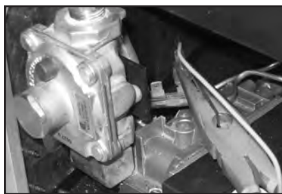
Figure 33: Spill Switch Wires Connect to Thermocouple.
