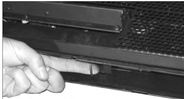
Figure 7: Adjusting the venturi air setting.
