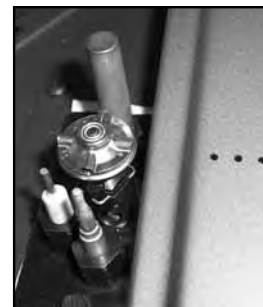
Figure 13: Ignitor assembly beside the burner.
