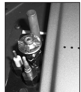
Figure 11. Ignitor assembly beside the burner.
