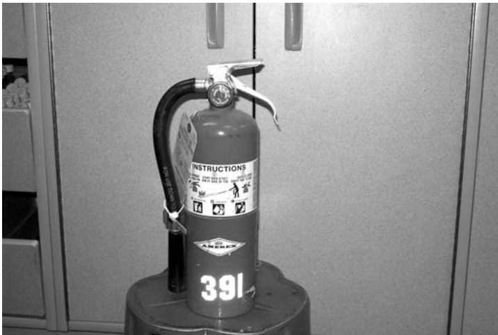
Figure 5-10 Portable extinguishers are marked to indicate what type of fire they should be used on.
