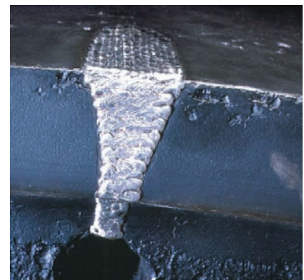
Low heat input and Xuper NucleoTec 2222 minimise residual stresses when performing massive repair welds on cracked cement kiln tyres.
