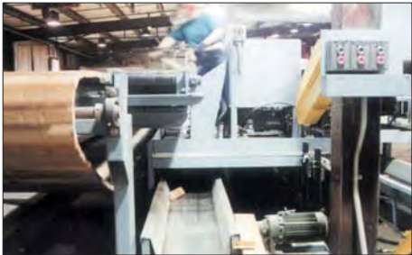
Once flooring is side-matched, it is inspected for defects. This conveyor, driven by Sumitomo Cyclo® drives, carries defective material to the hammer mill.
