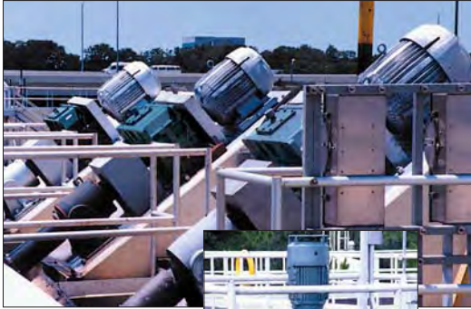
Each of these Sumitomo Paramax® speed reducers helps pump up to 13 million gallons a day at this state-of-the-art wastewater treatment facility in the City of Clearwater, Florida.
