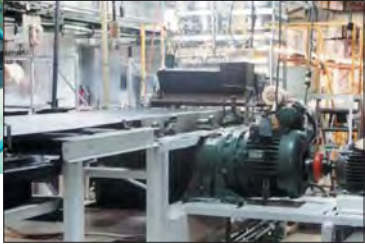
A 15-hp Beier mechanical variable speed drive with electric remote control provides an adjustable, steady speed range for this 350-ft. oven band conveyor.
