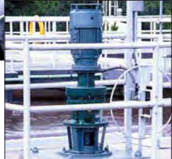
Cyclo® mixer drives are a key component of this award-winning water treatment facility in Hillsborough County, Florida.
