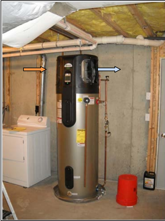
Figure 7. HPWH installed with adequate clearances
