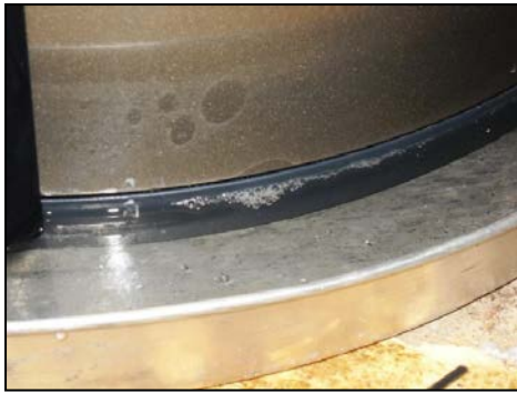
Figure 10. Condensate problems from improper installation
