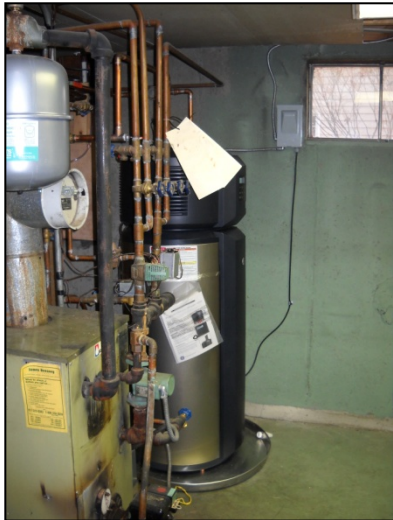
Figure 9. HPWH installed in boiler room
