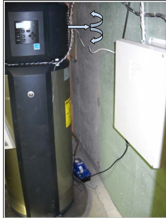
Figure 8. Improper HPWH with air discharge facing wall
